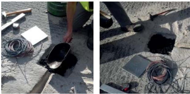
Road thermal sensors
